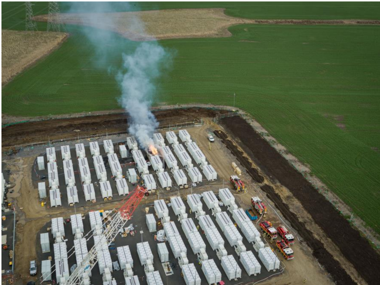
Figure 4 Victoria Big Battery fire incident [47]
