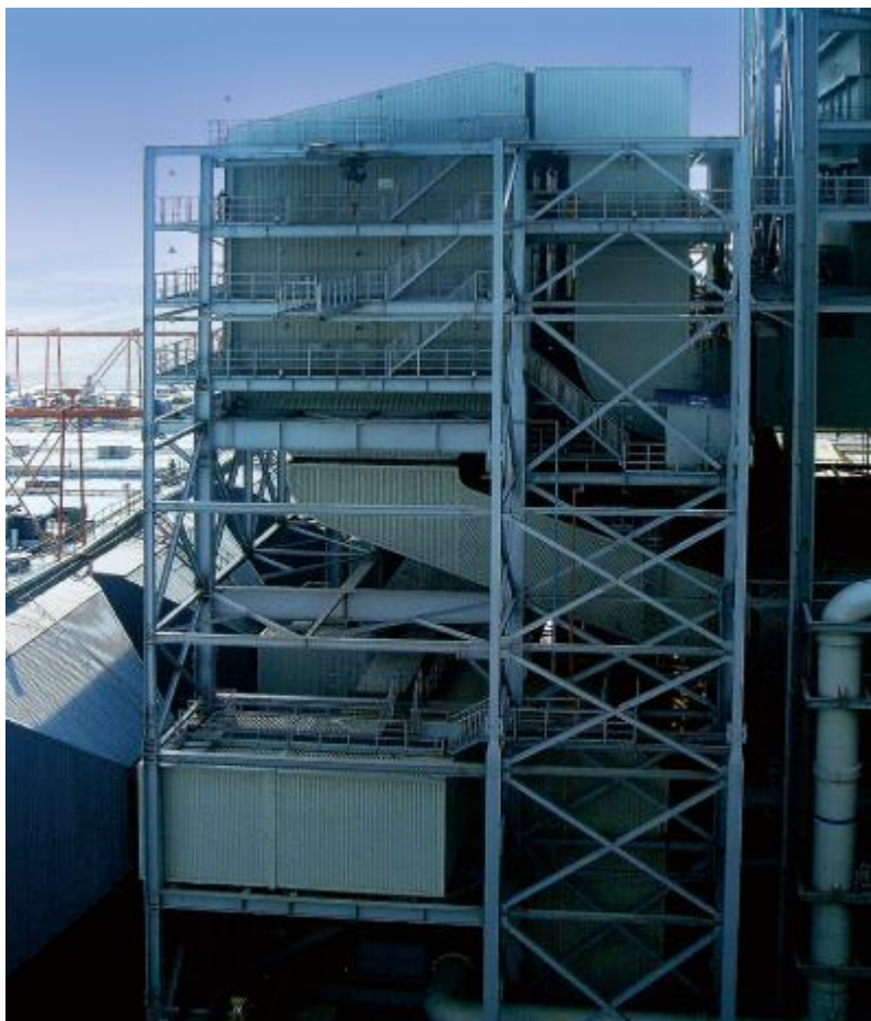
Figure 5.4 SCR system installed at a power plant (Zhejiang Feida Environmental Science & Technology Co., Ltd., n.d.)
