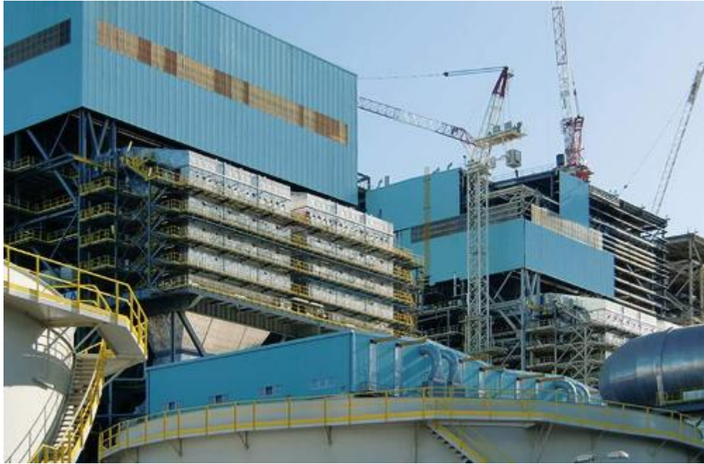
Figure 5.5. SCR systems at three 660MW steam generators (Steinmüller Babcock Environment, 2019)
