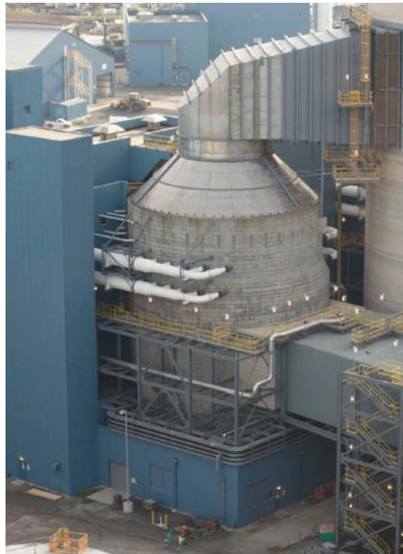
Figure 5.3 Wet FGD System installed at a power plant with one absorber per unit (Babcock & Wilcox, 2012)
